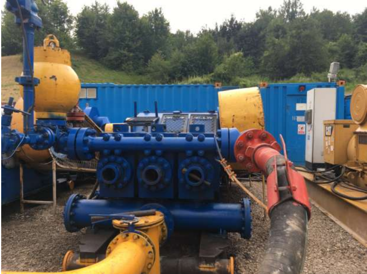
Figure 9: Mud pump in Foraj Sonde drilling rig in Draganeasa, Romania
